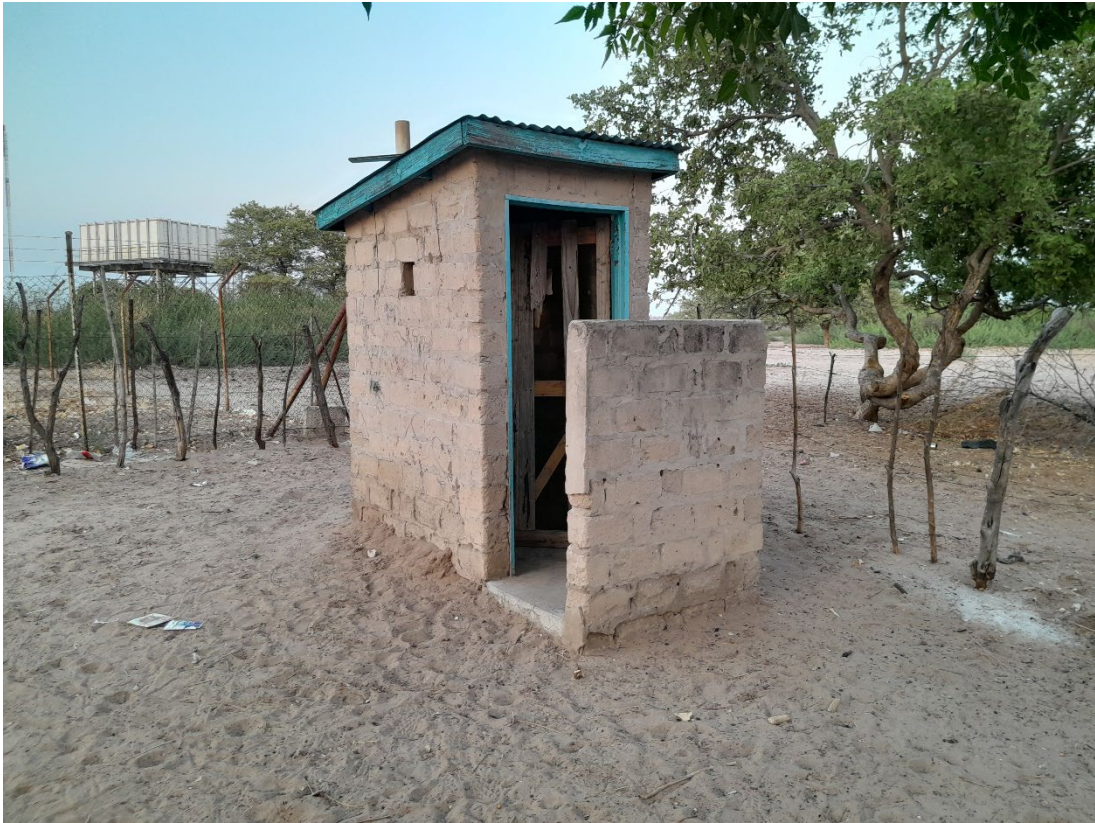
Photo 3: Toilet in New Xade Village (1).
